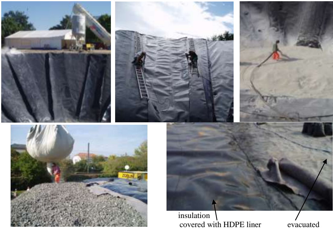
Fig. 6: Primary and secondary chambers, installation of the insulation by blowing from silo-truck into chambers or loose; lower left: installation of the foam glass gravel by pouring from big bags. It is delivered by trucks and filled on-site into the big bag by a front loader, lower right: filled and evacuated chamber.
