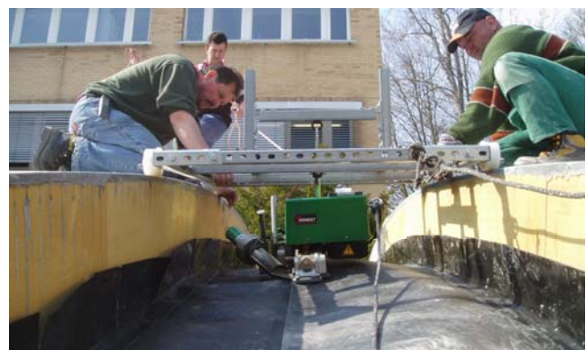
Fig. 6: Welding of the composite liner between two elements from the top of the cover
