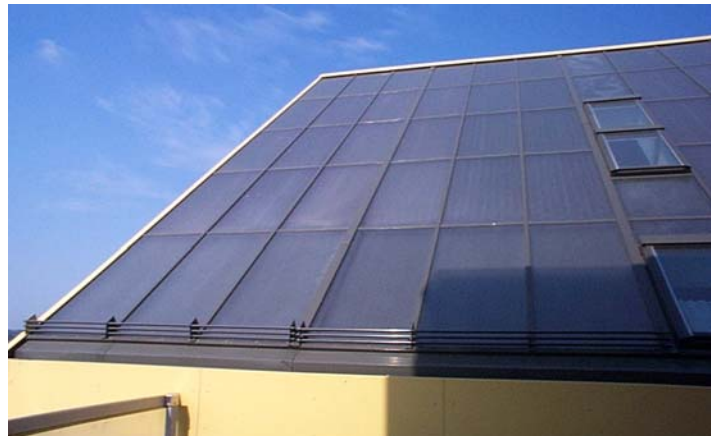
Figure 2: Solar roof with integrated windows and blind-elements without absorbers in temporarily shaded parts
