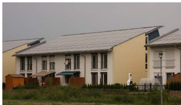
Fig. 9: Solar collectors on the terraced houses
